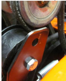
Bad - too close to pulley/belt
